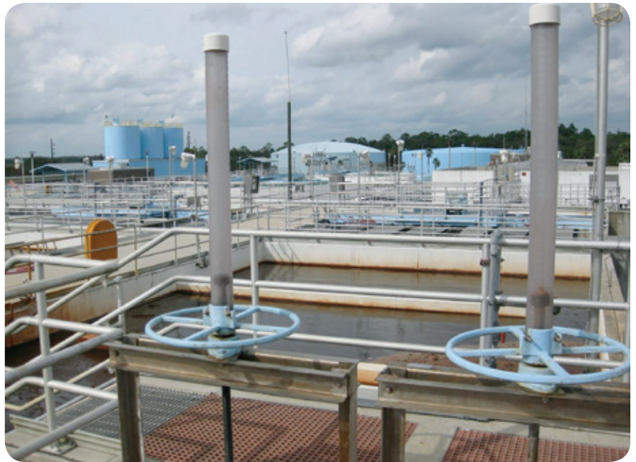
Dyal Water Treatment Plant
